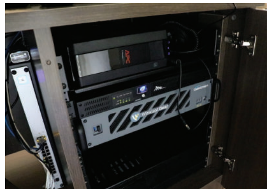
Wirecast Gear in rack
